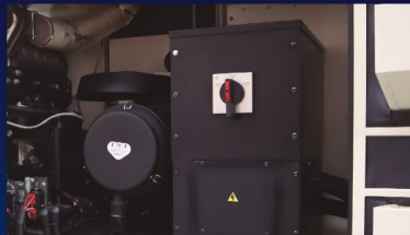
Switch Voltage Selector Mounted on a box above the alternator with automatic shut-off when the door is opened.
