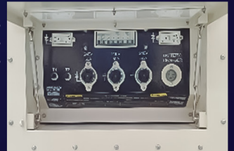
GFCI Outlets Electrical Twist locks Flange outlets Minibreakers for control
